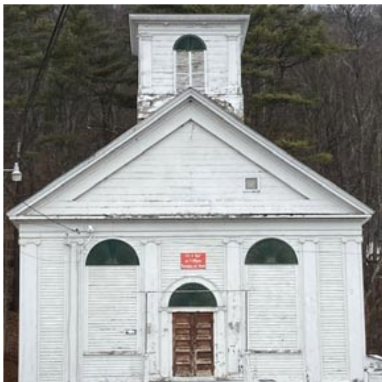
Shown in a recent photo, Bradford's 226 year-old "old church" is now owned by Old Church Theater Inc, a non-profit community theater organization. Plans are underway to renovate it into a year-round performance center.
